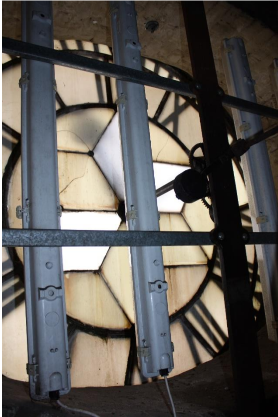
Another view of a dial, showing poorly replaced opal panels, and extensive corrosion to the iron tracery, and cracking to older glass panels.
