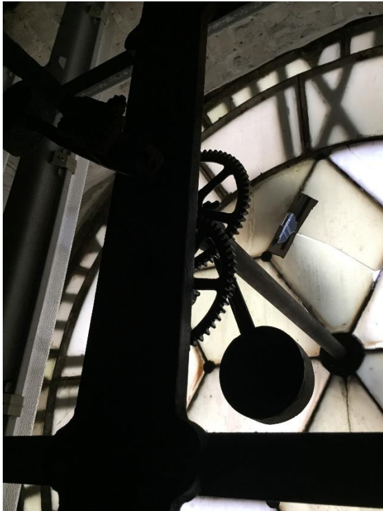
Many opal panels are cracked and broken, rust is widespread, and some panels have been replaced with unsuitable acrylic in the wrong colour.
